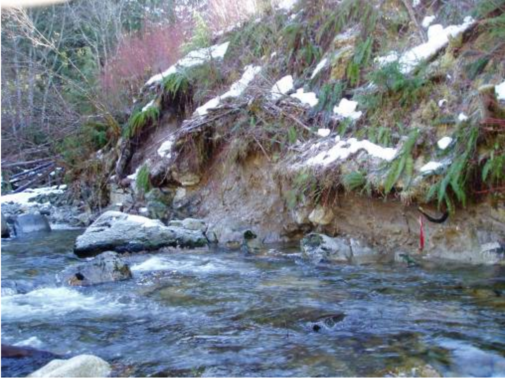
Appendix Figure 3. Reach-1 656 m steep riffle: 2 parallel rootwads off left bank using local ballast boulders, for erosion control on BCH power-line right-a-way.
