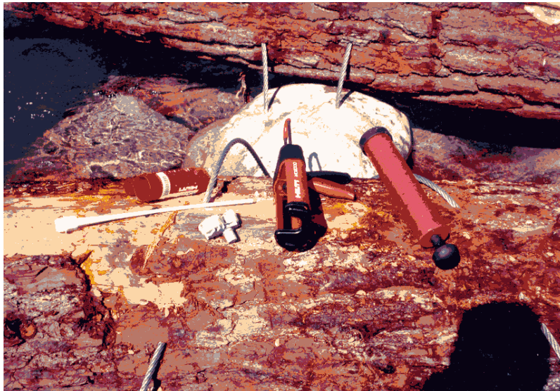
Figure 7. Example of cabling of triangular rootwads using Hilti epoxy to secure LWD to boulder ballasts (with left mid-cable not yet inserted).
